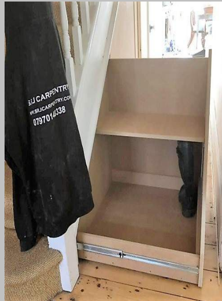
Under stairs drawer storage unit.
